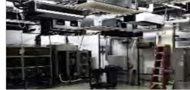
LG Air Conditioning Academy
